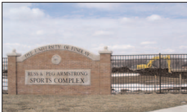
Construction is underway at the Russ and Peg Armstrong Sports Complex at the corner of Trenton and Blanchard. Ground has been broken for the new tennis courts.
